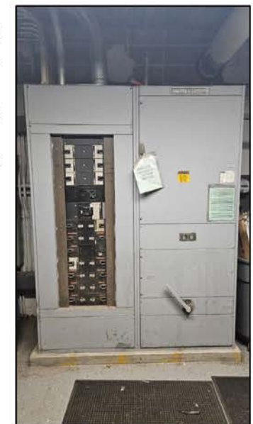
Figure 2: Existing Main Switchboard in Maintenance Room
