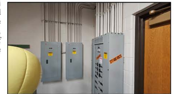
Figure 6: Distribution Panels in Storage Room
