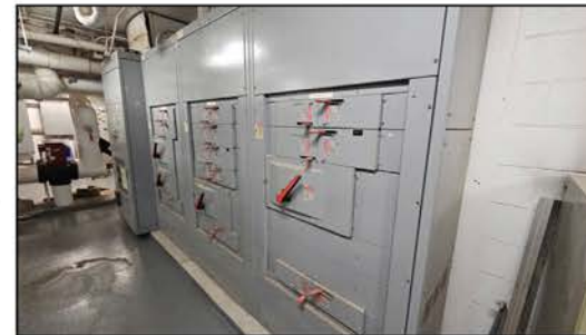
Figure 2: Existing Main Switchboard in Boiler Room
