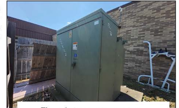
Figure 1: Outdoor utility transformer
