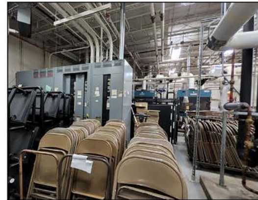
Figure 2: Existing Main Switchboard in Boiler Room
